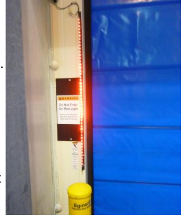
VIRTUAL VISION ALERTS PERSONNEL TO APPROACHING TRAFFIC WHERE THERE IS OBSTRUCTED VISIBILITY
