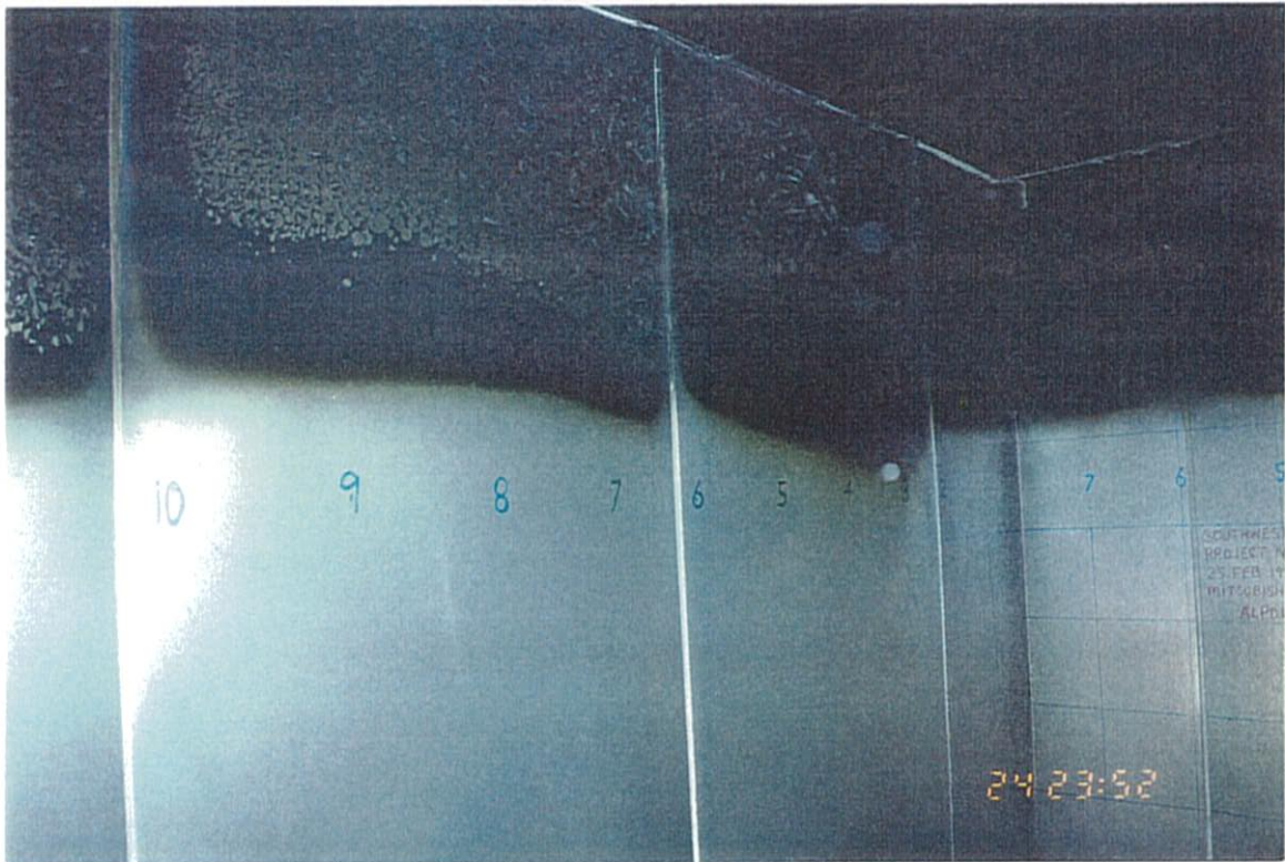
Figure C-3. Room Interior Showing Left and Back Walls. Note blistering and flaking of paint coating on aluminum skin.
