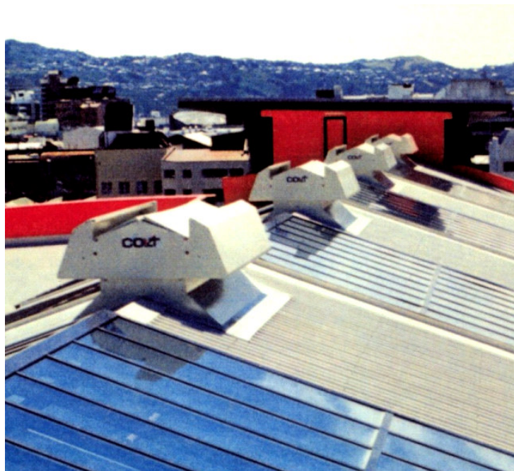
Colt MF/MMF/0924 Ventilators installed in the Atrium Roof of School of Architecture, Wellington.
