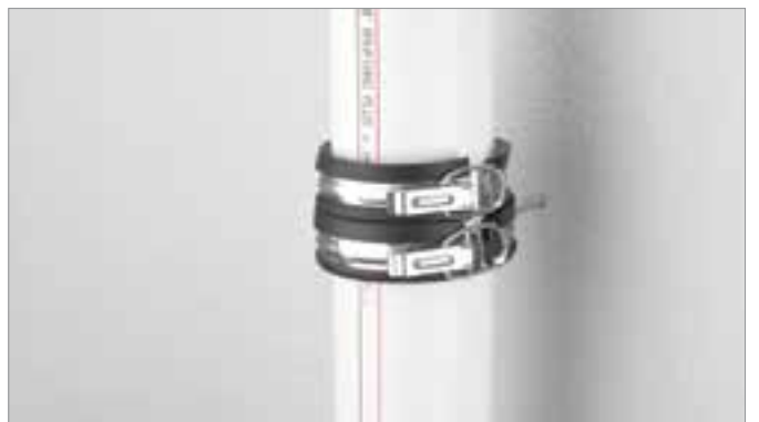
Fig. 7-17 Fully installed sound-dampening bracket.
