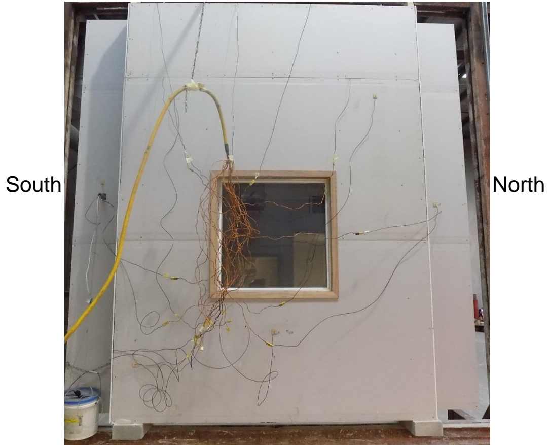
Figure A6.3: Unexposed face of specimen at the end of the test
