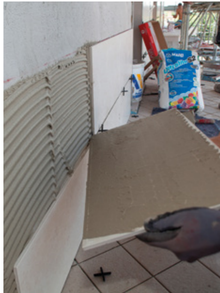
The correct method to install tiles on a façade using the double-buttering technique
