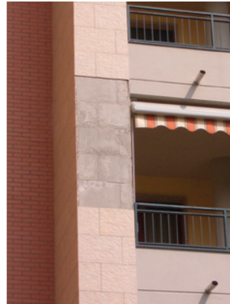
Detached ceramic installed on a substrate without joints
