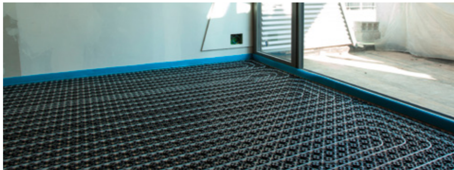
Substrate with an underfloor heating system
