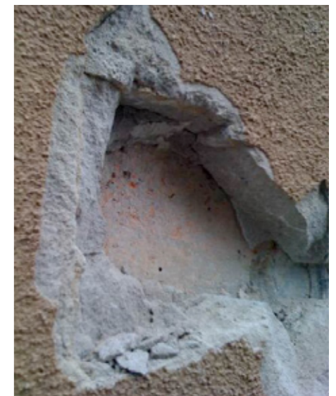
Failure of render unsuitable for bonding ceramic
