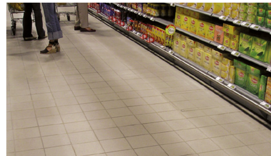
Floor in a supermarket subjected to stresses and loads from the constant passage of concentrated loads that requires the full wet bed installation method
