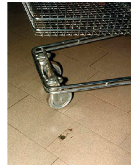
Tiling damaged by a concentrated load
