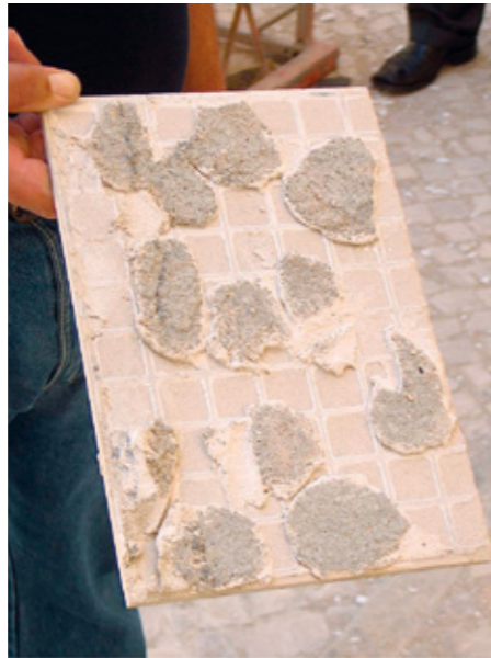
Tile detached from a substrate due to incorrect application of the adhesive (spot bonding)
