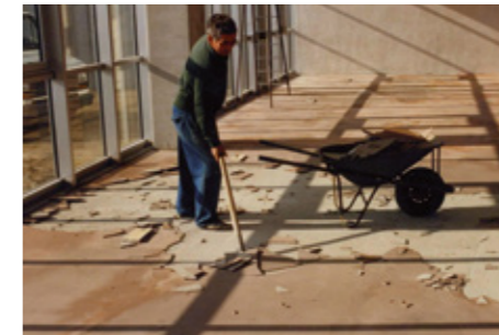
Detachment of a skim coat on a screed with irregular areas of strength
