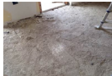
Substrate unsuitable for installing ceramic
