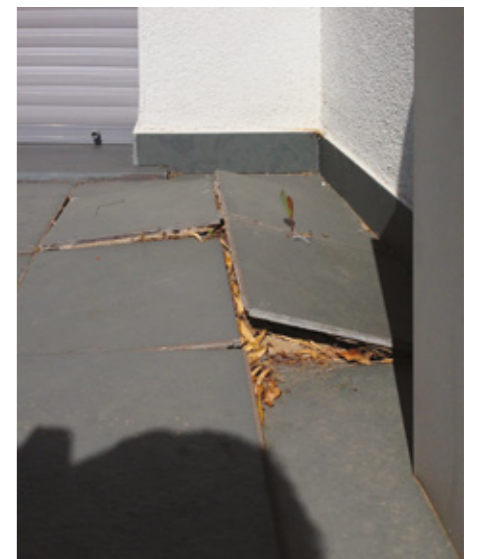
Detachment caused by compressive loads acting on an external floor due to a lack of joints
