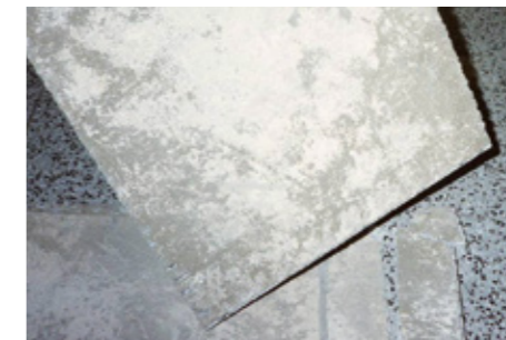
Tiling detached due to poor cleaning of the substrate
