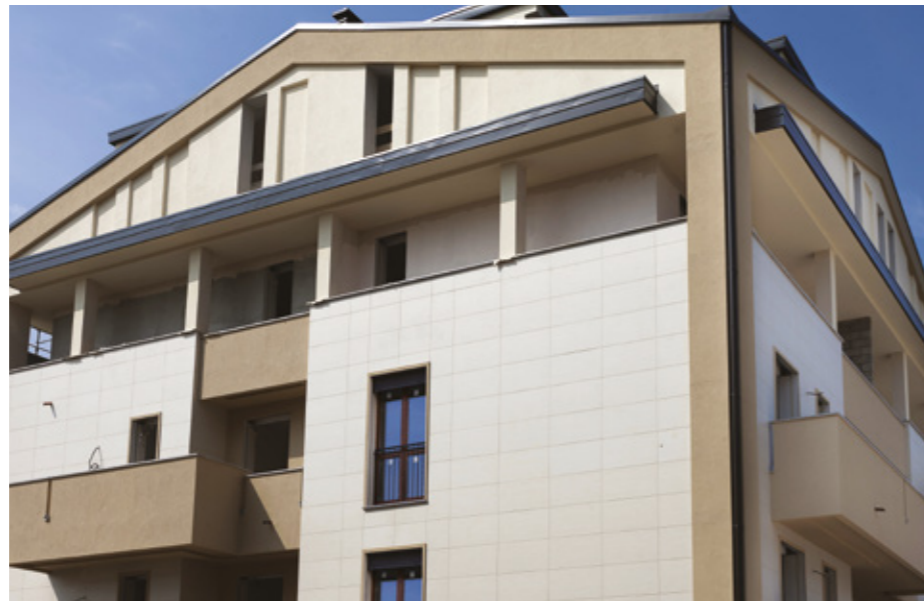
Installing tiles on surfaces exposed to sunlight using deformable adhesive (optional class S1-S2)
