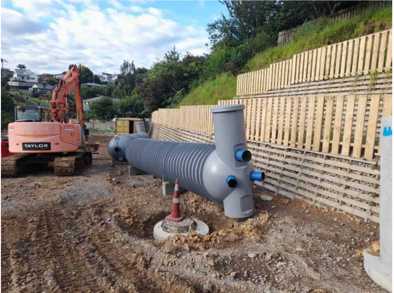
2x 10,000L end to end - multiple welded connections
