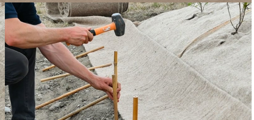
Drive poles to 250mm above ground using the pilot pole as a guide
