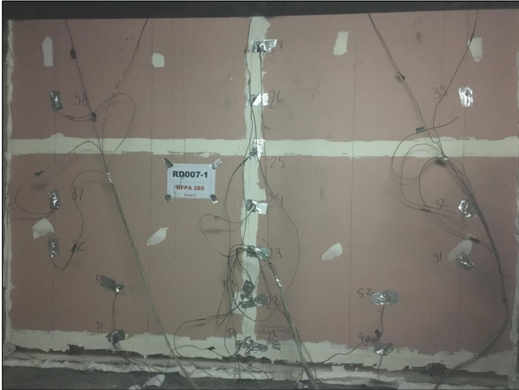
Picture 15: The interior of the base wall in the second floor test room at the end of the test.
