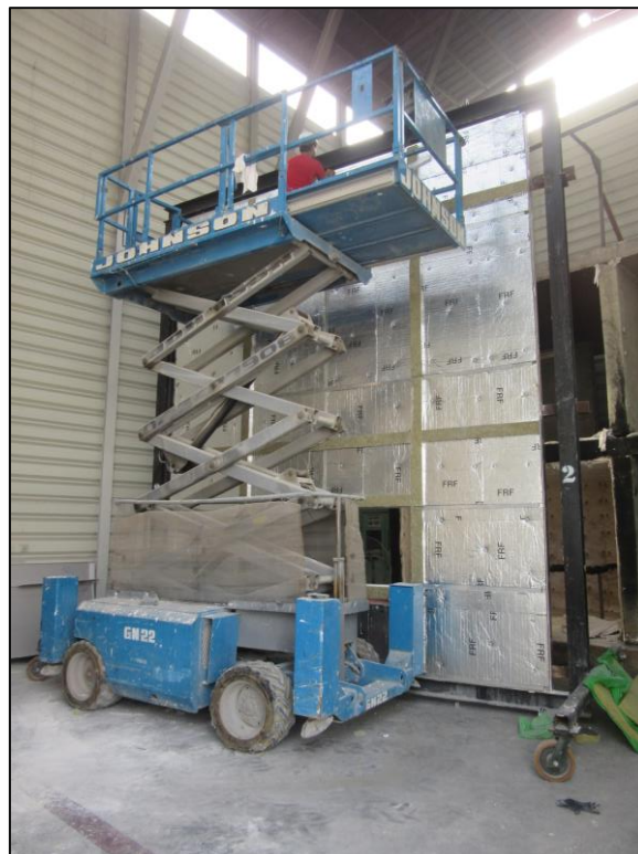
Picture 4: External insulation and cavity fire barrier fixed over the base wall.
