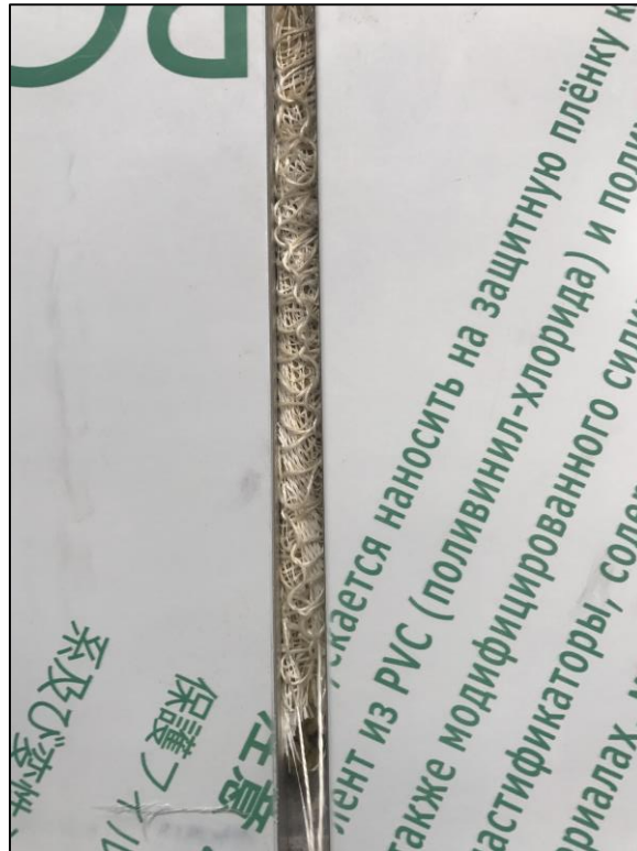
Picture 9: Firestop rope backer rod fitted into the gap between the panels.
