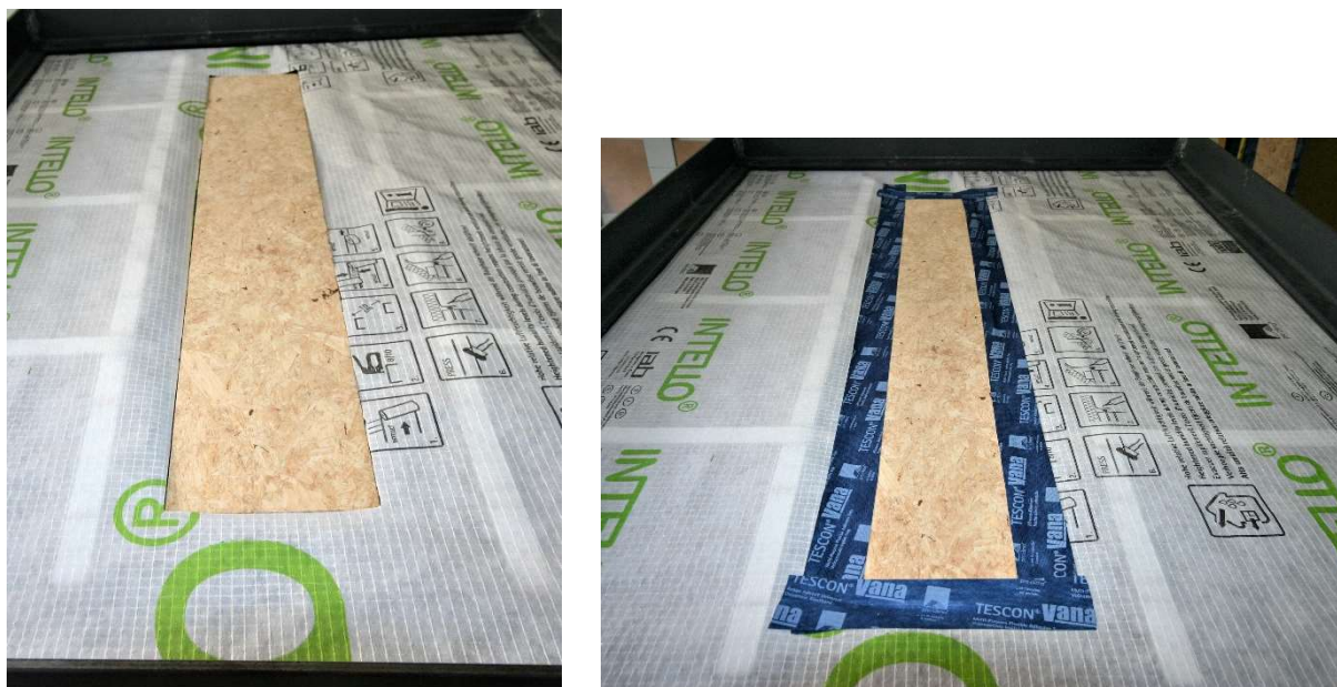
Fig. 2: Cut out membrane with OSB panel (left). OSB panel joined to the membrane on all four sides using TESCON VANA (right).
