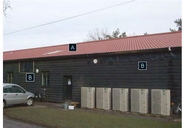
A: Vent cut in roof by fire service. B: Vents cut in wall by fire service.
