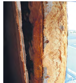
Window removed by Fire Service to ventilate the building to gain access – no fire penetration of core material.
