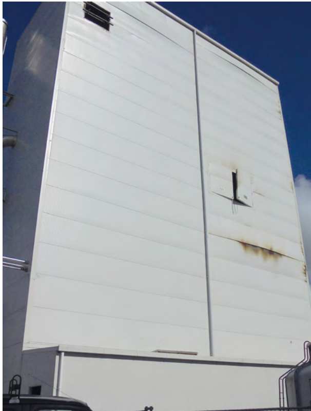
Milk powder drying tower showing external fire damage to panels (explosion doors opened manually after fire).
