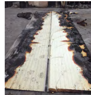
Panel at junction with steel stripped off demonstrating charring of PIR core but no evidence of fire spread.
