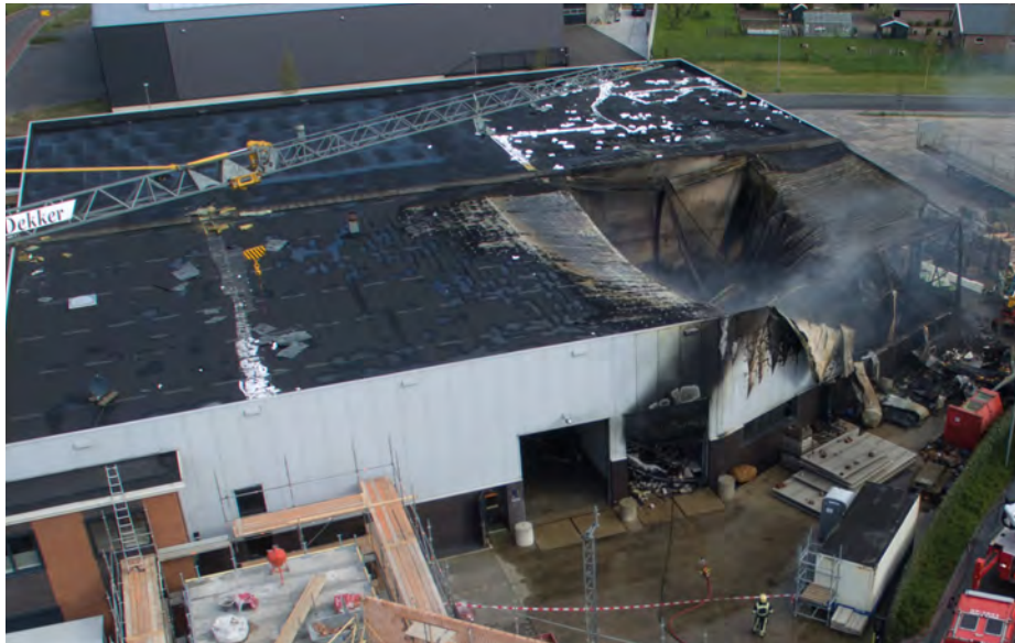
Aerial view of the damage showing structural collapse of the army surplus warehouse.
