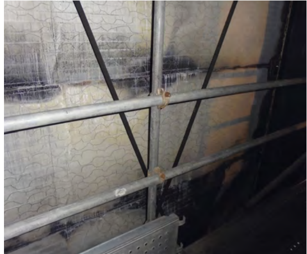
Panels exposed to fire internally.
