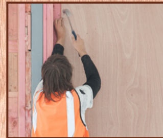
Economical Rapidline Okoume provides a simple, clean look. Left and above: Wall linings going up, private museum, Waikato.
