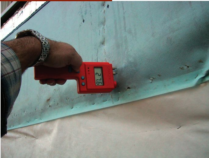
Low vapor permeable housewrap with high moisture reading on OSB under housewrap
