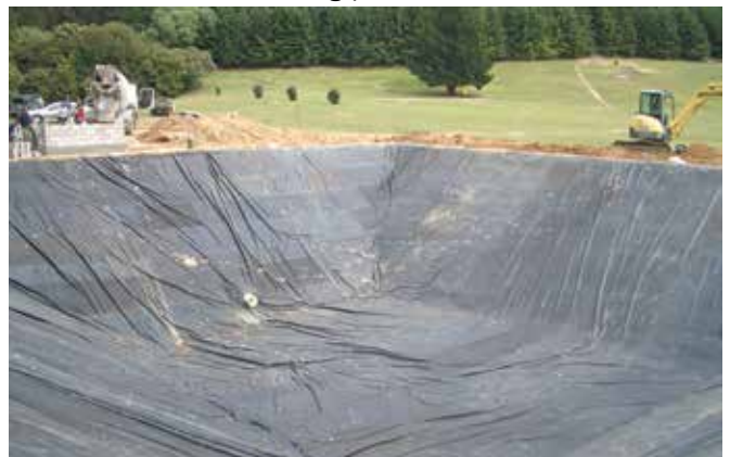
Storage pond for a golf club sprinkler system
